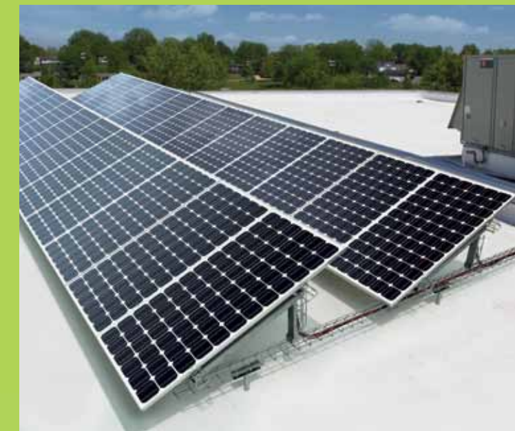
Angle support hardware and Delta Strut framing supported by roof stanchions.
