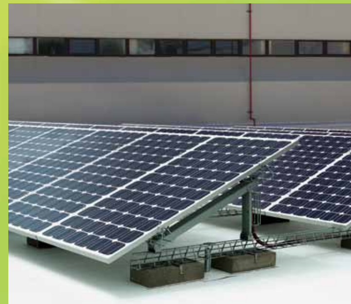
Angle support hardware and Delta Strut framing attached to concrete ballast blocks and roof stanchions.
