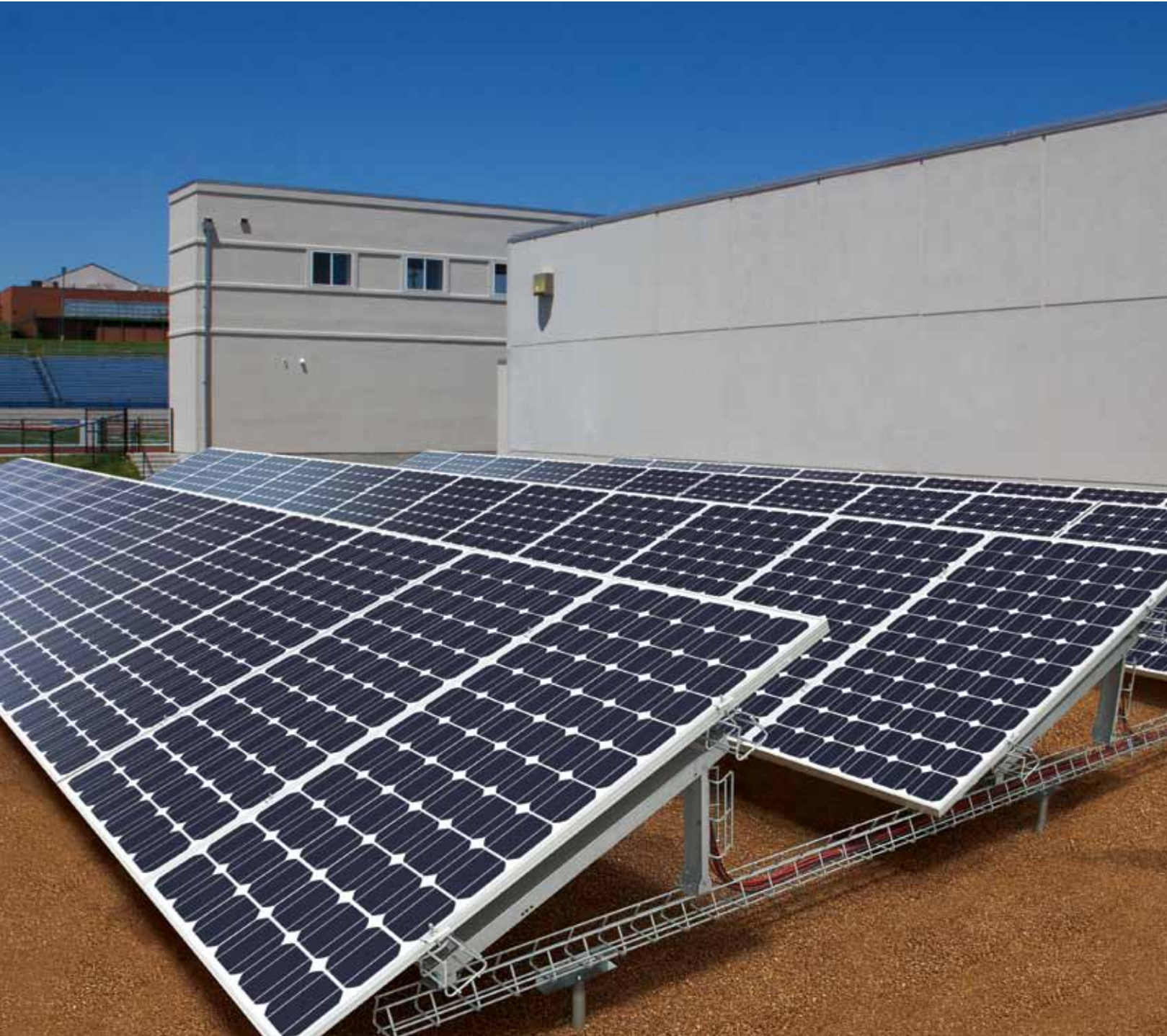
Angle support hardware and Delta Strut framing supported by roof stanchions.
