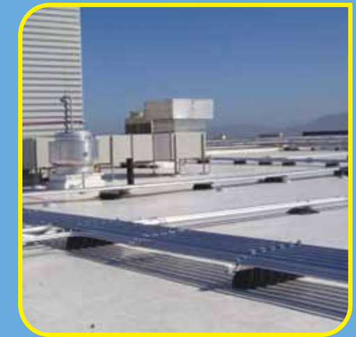
A clean and orderly rooftop installation can enhance building value.
