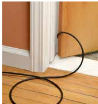
Inappropriate use of extension cords, such as placement under rugs or in a door jamb, can result in damaged conductors.
