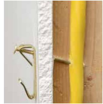
A drill bit or nail can sever the insulation of cable inside a wall.
