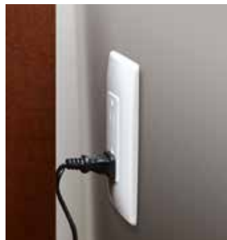
Furniture pushed against the plug of an appliance cord can stress conductors and damage insulation.
