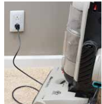
Wear and tear of appliance power cords can eventually lead to damaged conductors.
