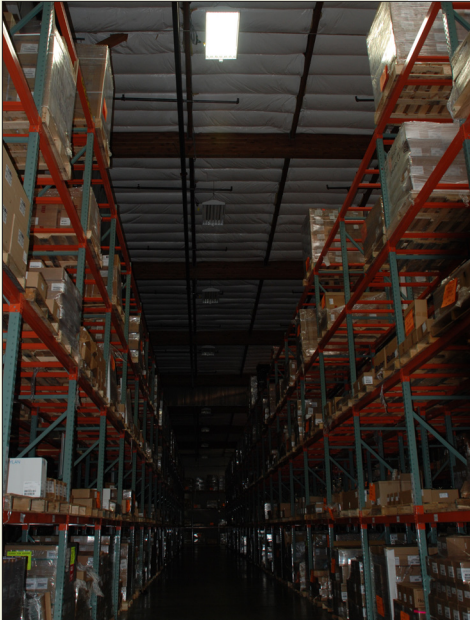
Occupancy sensors turn on individual lights as needed and turn them off following a time delay.
