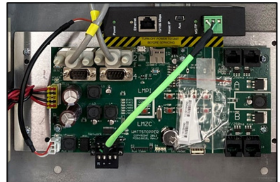
LMPI board with both cables attached
